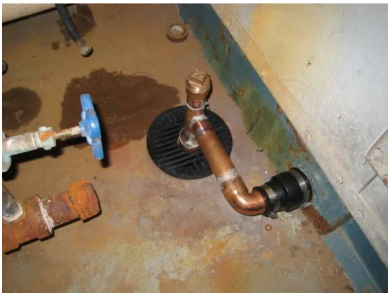
Concentric Trap installed at Smithsonian Institute
